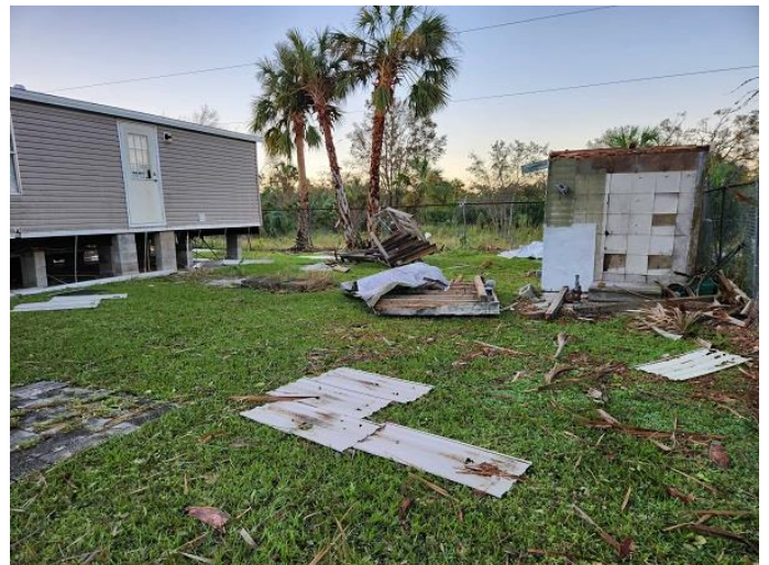
The staircase was ripped off the 1996 unit and its skirt sections everywhere. The roof of the c. 1975 newly-remodeled mower shed lies beside it.
